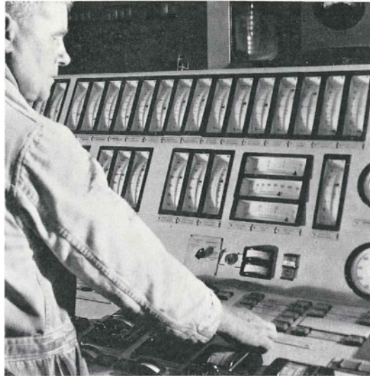
Boiler drum water level presentation
